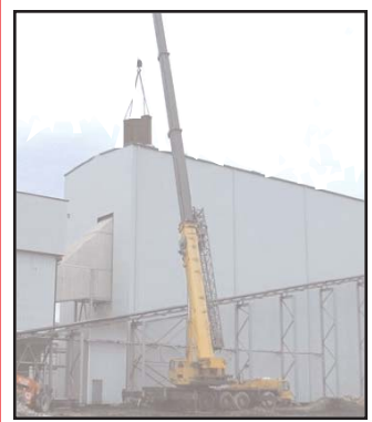
This photo shows the "Steam Economizer" equipment being hoisted into position by the crane on March 14th..
