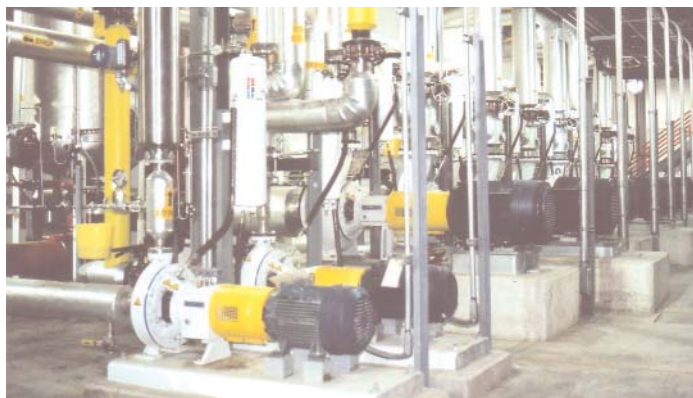
Water is “pulled” out of the thin stillage to create syrup using the equipment of this efficient evaporator system.
