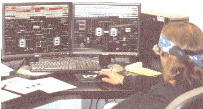
Control panels like the one above in the Plant Control Center serve as the “Nerve Center” for the entire plant.
