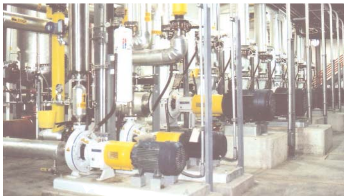
Water is “pulled” out of the thin stillage to create syrup using the equipment of this efficient evaporator system.
