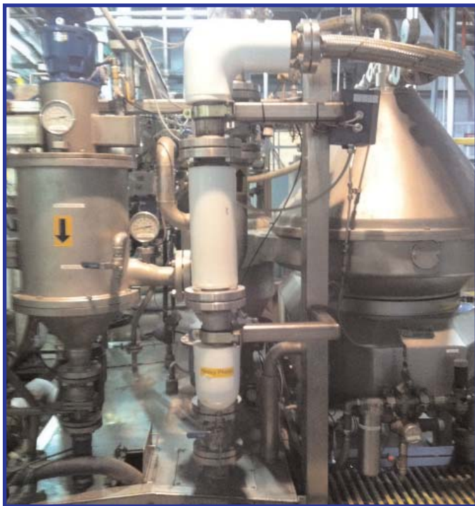
This is a picture of the oil separation equipment.
