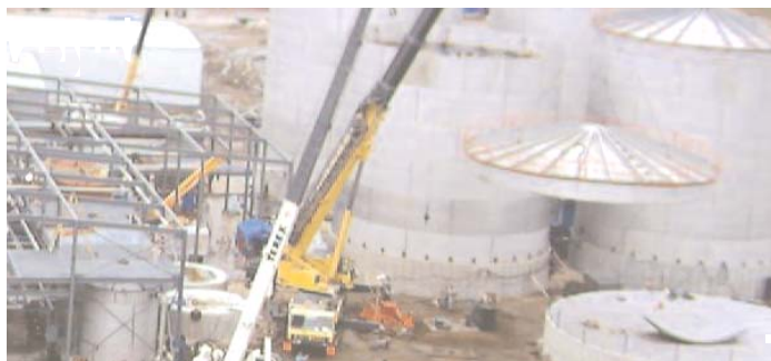
A crane lifts a lid into place on one of the four 760,000 gallon fermentation tanks on August 11th
