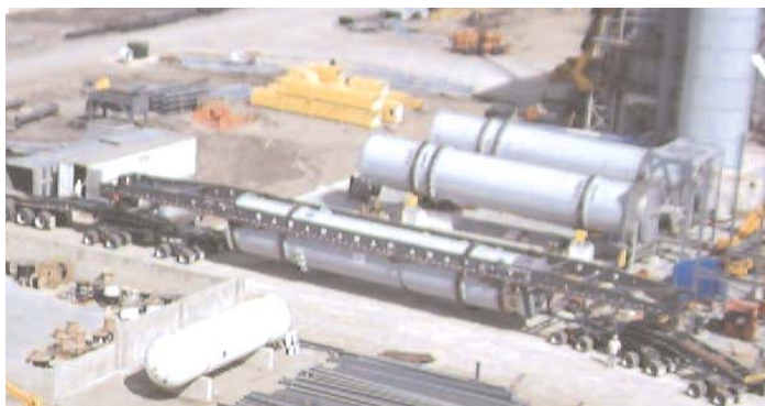
On September 22nd a specially built tractor trailer rig transporting the third steam tube dryer arrived on the site, ending a two day long, 450 mile journey of a rig that measured 300 feet in length to handle this equipment.
