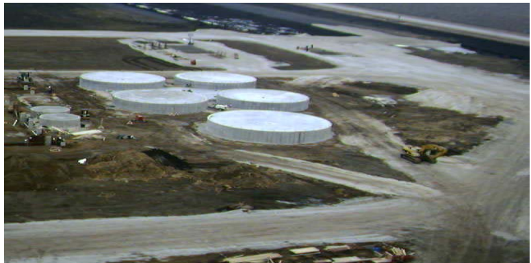
Fermentation tanks and beerwell located on the south side of the plant. Processing Building will connect on the left side and run through the center of the 4 tanks. Photo taken 3/25/05.
